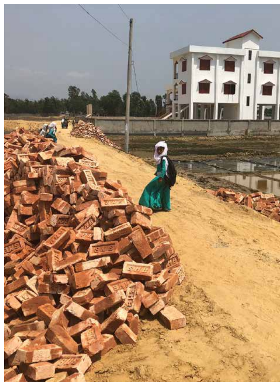
One of eight rural roads built by 100 volunteers as part of a cash for work programme in a host community close to the Rohingya refugee camps. The raised roads benefit families walking to their fields, children going to school, livestock grazing and enables small transport vehicles to reach resident's homes and livelihoods. Photo: Stacey Winston\UNDP
