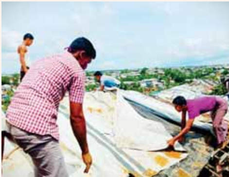
A disabled person is being helped to repair his house rooftop as part of monsoon disaster preparedness. Photo: Alam
