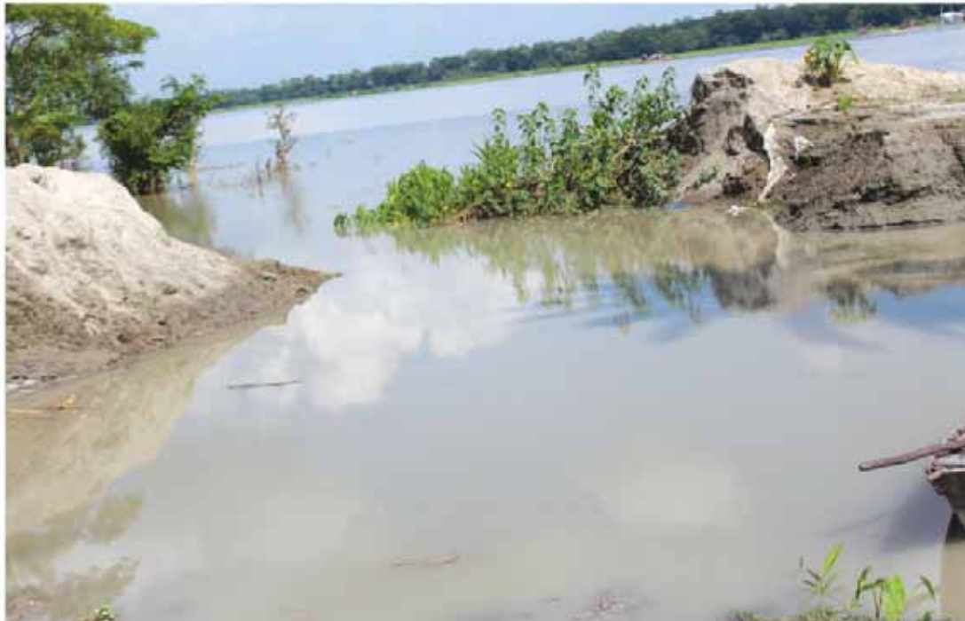
The damaged embankments have not been repaired yet as a result saline water is entering the locality with the tide and increasing the economic loss to the local community. 7 no- ward Fedai Nagar, Jain Kathi Union, Patuakhali.
