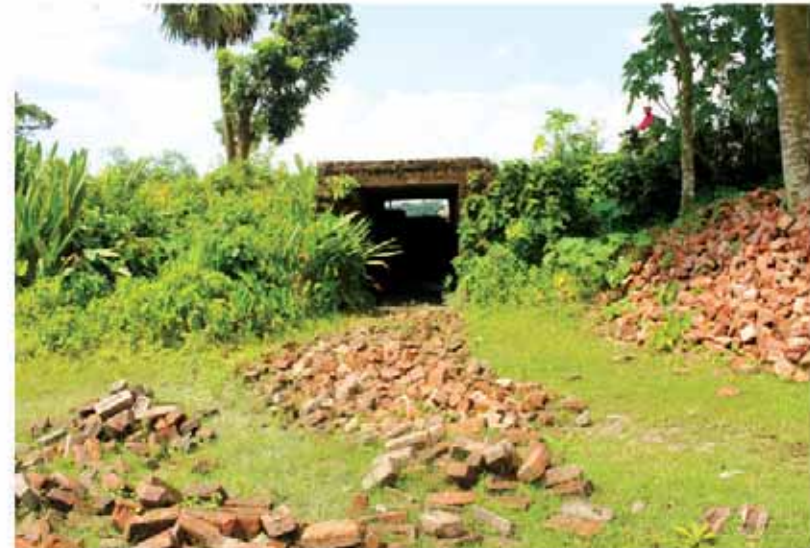
Several Culverts in various important places of Jainkathi Union have been completely or partially damaged due to frequent natural disasters Photo Credit: Jainkathi Union
