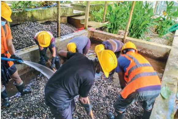
Faecal Sludge Management, Rohingya Refugee Camp 15, Ukhiya, Cox’s Bazar, Bangladesh. Photo: COAST Foundation Archive
